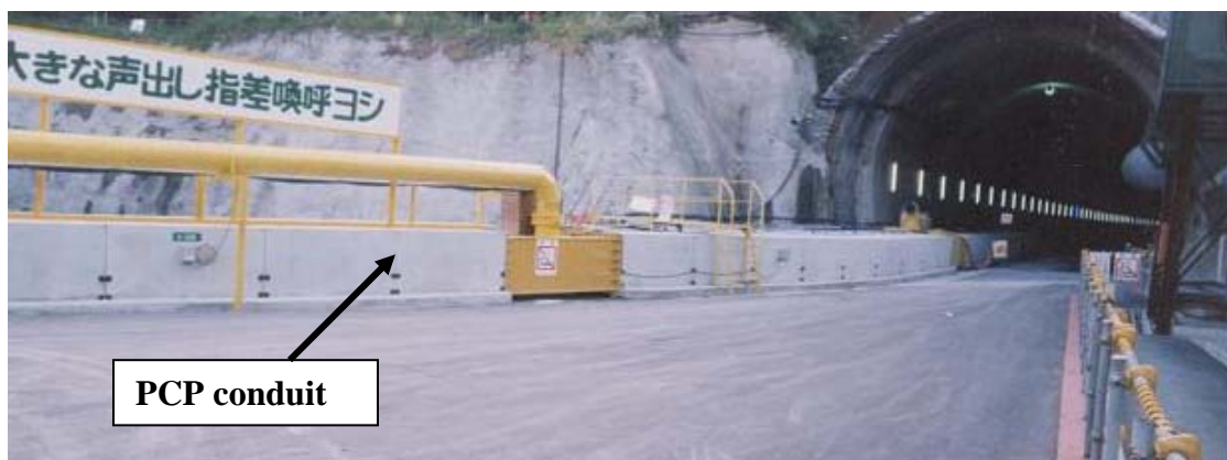
(a) PCP conduit entering/leaving the Tunnel
